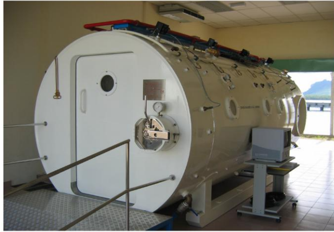
Fig 9: Typical installation of HBOT
