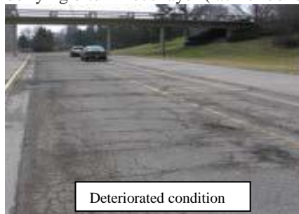
Fig-2: Deteriorated condition pavement surface
