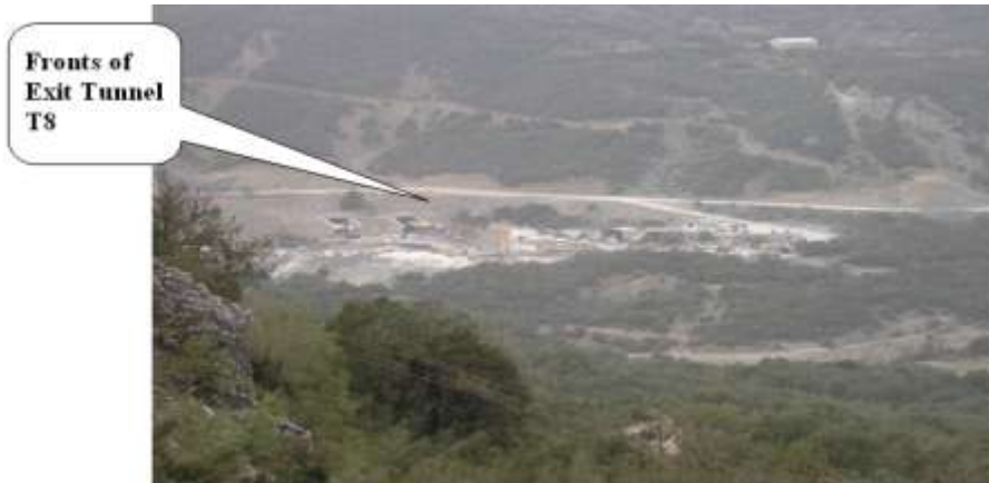
Photo 1: Area A (Fronts of Exit of the Tunnel T8 of Egnatia Highway).
