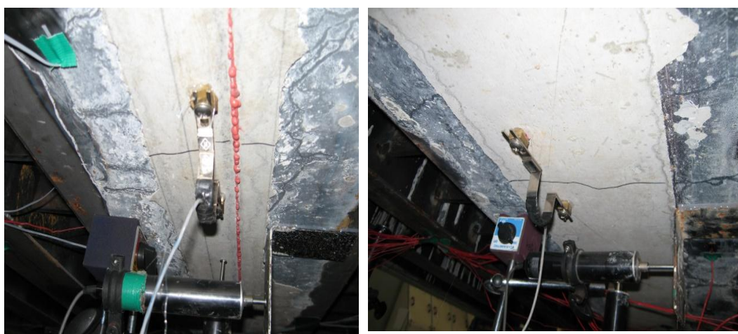
(a) Deck specimen with mechanical joint (JD9B-F) (b) Deck specimen with lap-spliced rebar (JDLS-F)
