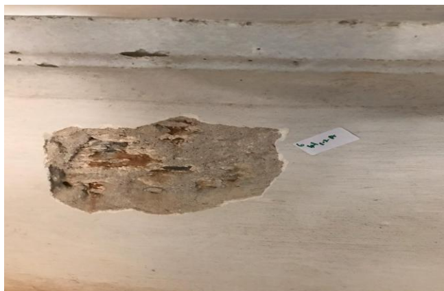
Fig. 1 Deterioration due to spaling of mortar
