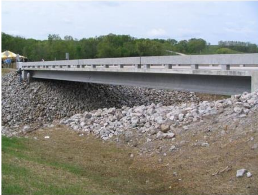
Figure 1. This Wapello County, Iowa structure was the first UHPC bridge constructed in the United States.
