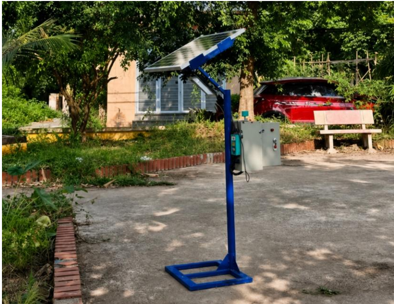
Fig. 3. Outdoor installation of the developed solar lighting and monitoring prototype.
