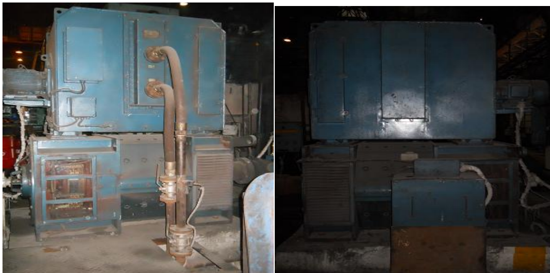
Fig 5 – cooling system of 600 kW DC motor.( with circulating water with inlet and outlet vent.)
