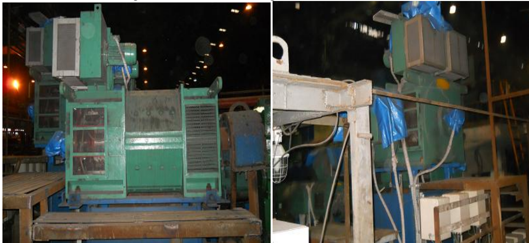
Fig 3 – cooling system of 600 kW DC motor. Forced air cooling
