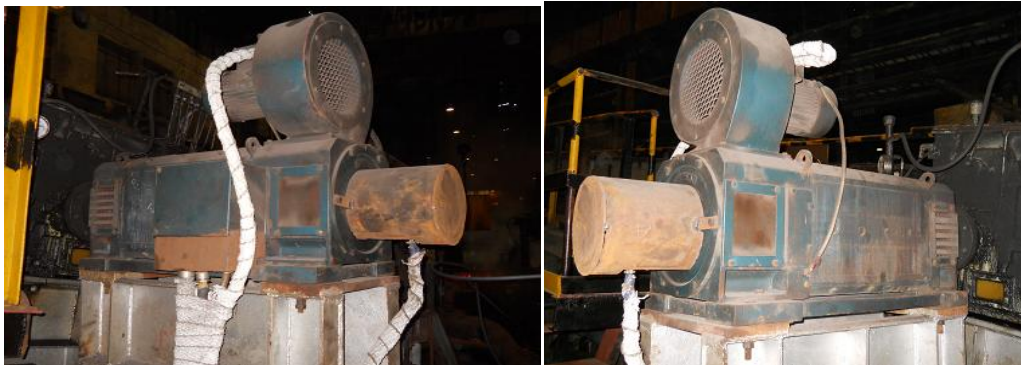
Fig 2 – cooling system of 75 kW DC motor. Forced air cooling
