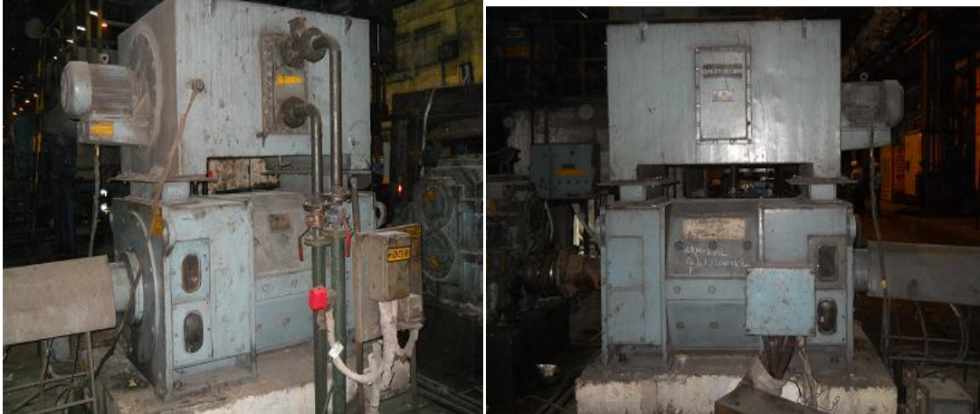
Fig 4 – cooling system of 600 kW DC motor.( with circulating water without inlet and outlet vent.)
